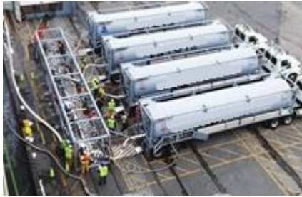
Figure 4.11 – LNG bunkering with multiple trucks, via common manifold
