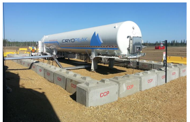
Figure 12.8 – LNG trailer semi-fixed installation. Despite not being a purely TTS bunkering operation it gives evidence on how felxible LNG trucks and trailer can be. Here a semi-fixed installation that may be used for LNG bunkering or fuelling. Typically an installation for LNG consumption more than bunkering/transfer.
