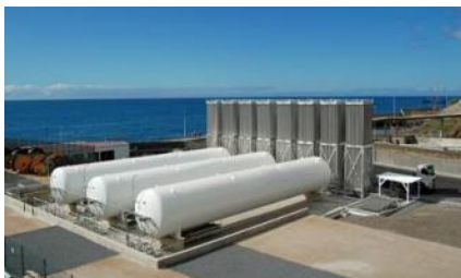
Figure 4.13 – Small scale LNG storage – pressurized tanks and evaporators for re-gasification.
