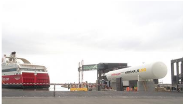
Fig.2.9 – Fixed LNG bunkering facility, with small-scale LNG storage tank.
