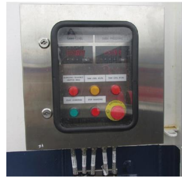
Figure 2.47 – ESD local command switchboard and alarm indicator [26]
